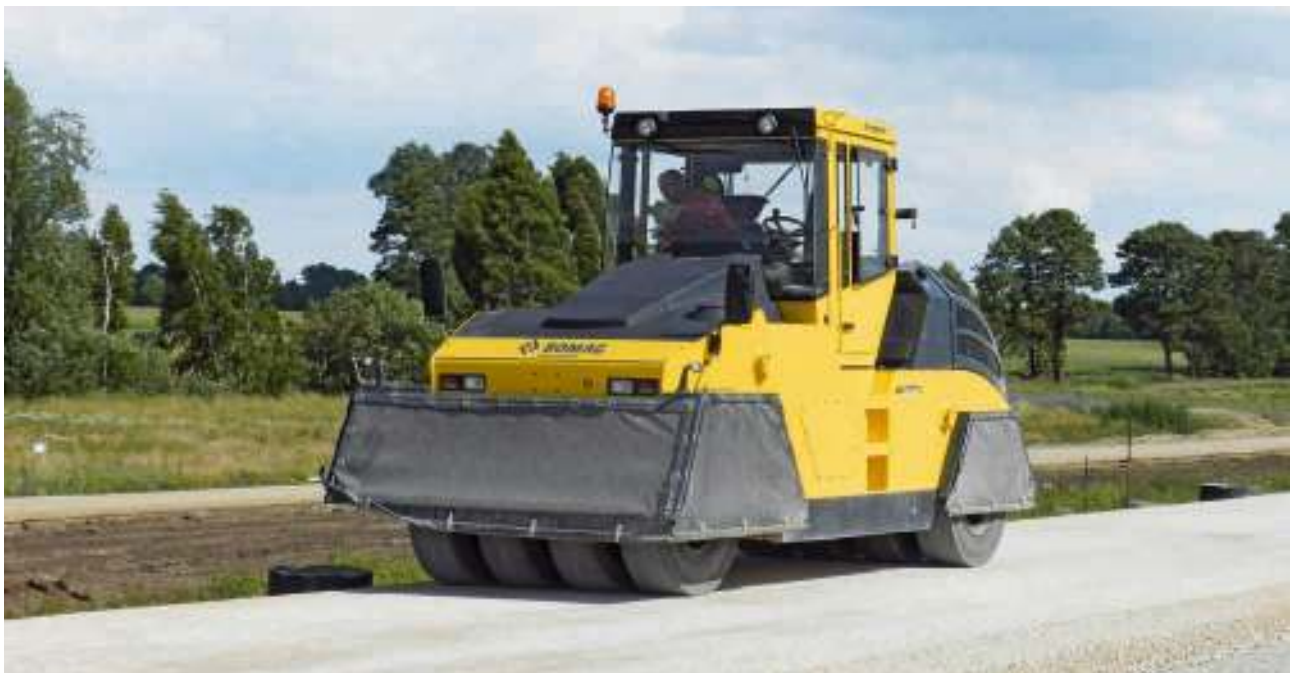
BOMAG pneumatic tyred rollers are also used for earthworks compaction and surface sealing.
