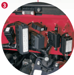
Electrical fuse box and relays
