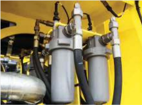
Discharge side of the hydraulic filter system.
