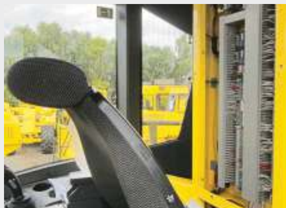
Well protected control centre in the cab.
