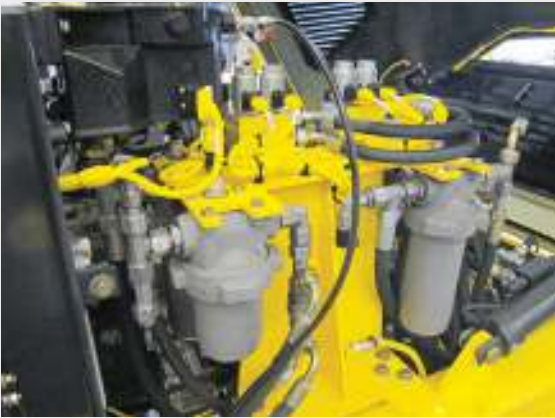
Discharge side of the hydraulic filter system.
