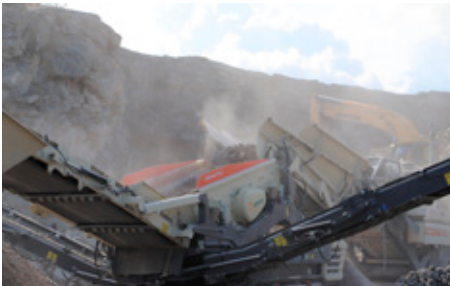
Multi-use for primary scalping and screening.
